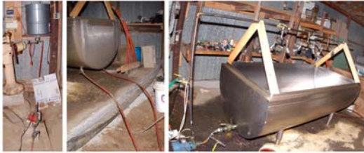
Above: The new drier (right), PEX tubing in and out of the trough (center), and the pump and temperature monitoring (left).
